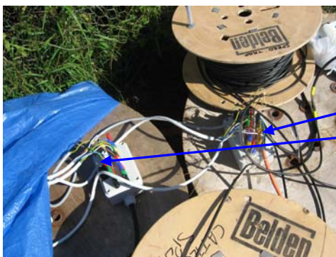
Multicore cables joined together
