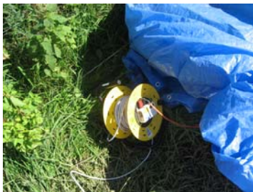
Cable to Radio Trans unit located by multicore cable drums
